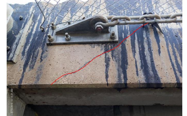
Figure 1. Typical appearance of diagonal crack on front beam, marked in red for visibility. Note that the crack shown does not appear to originate at the supporting element.
