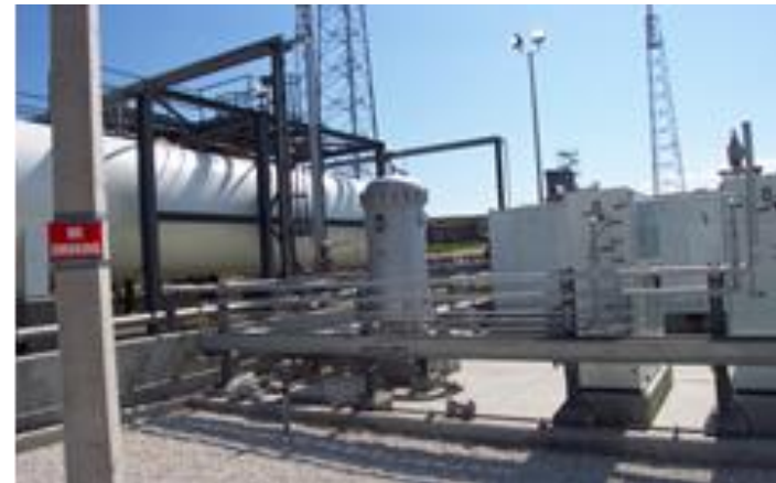
SLC-41 LH2 VJ Horizontal Storage Tank
