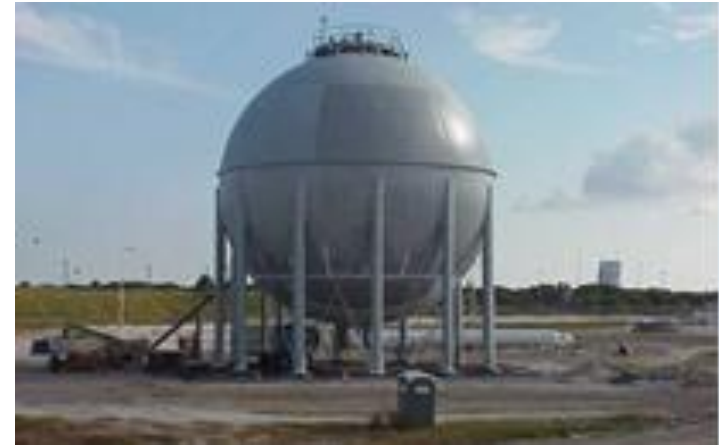
SLC-41 LO2 VJ Storage Tank
