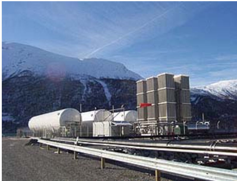
Figure 2-4 LNG receiving and storage terminal (Source: MARINTEK)
