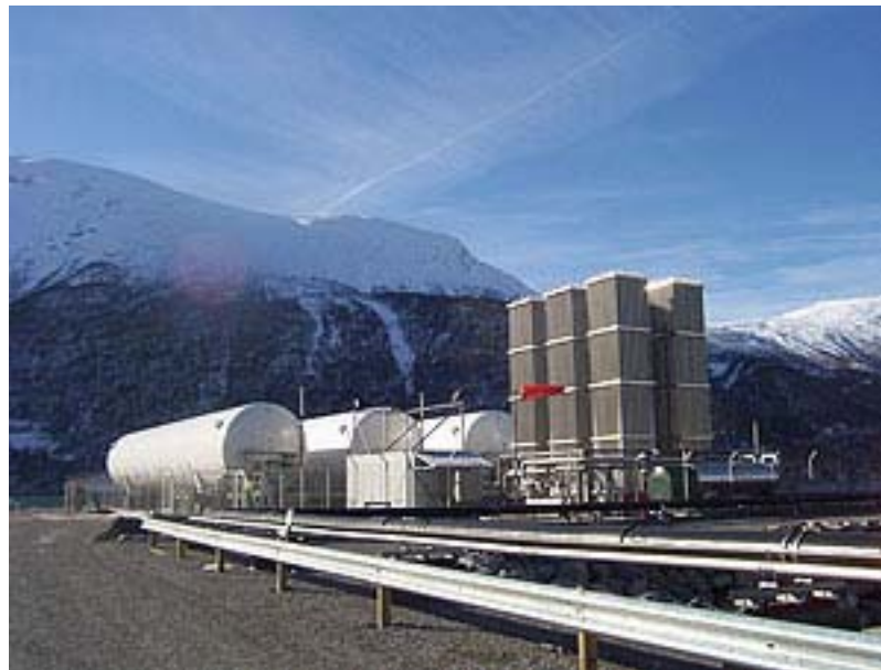
Figure 11-3 LNG receiving and storage terminal (Source: MARINTEK)
