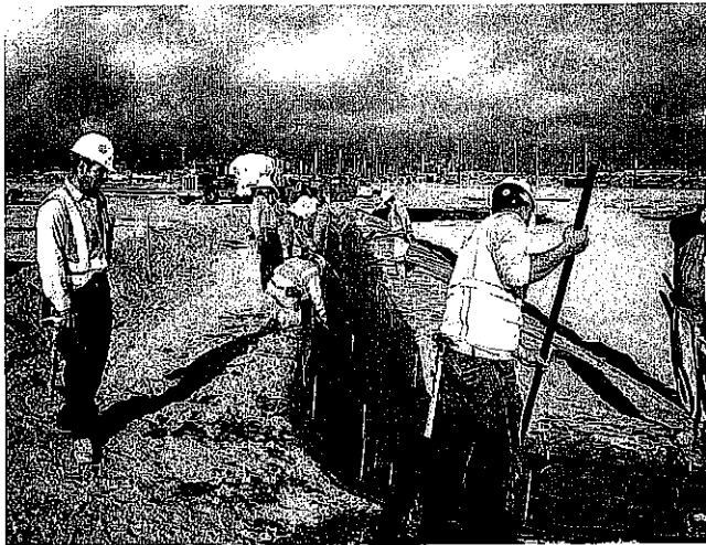
Construction of the collection v-ditch around one of the three detention basins
