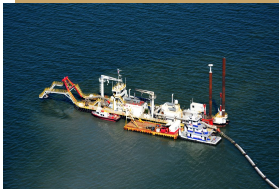
Manson Construction – Robert M. White Cuttersuction Dredge (30-Inch) Halimar Shipyard, LA - $40 M. ( Delivered )
