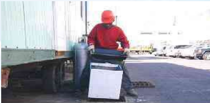
A worker inserts a catch basin insert for oil and grease, trash, debris, and sediment removal from stormwater as it enters the storm drainage system (Source: Ab Tech Industries, 2001)
